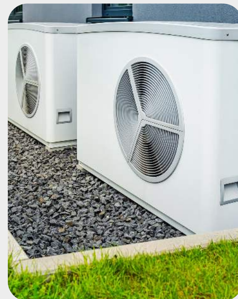
Air source heat pump
